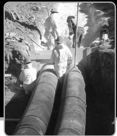
NATIONAL CENTER THERAPEUTICS MANUFACTURING - TEXAS A&M 24" HDPE CWSR INSULATED WITH GILSULATE®500XR. A&M'S CAMPUS DISTRIBUTION MASTER PLAN FOR CWSR/HWSR RECENTLY CHANGED FROM PIP TO GILSULATE®500XR.
