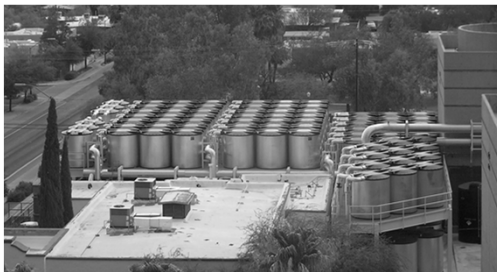
Ice Storage Tanks
