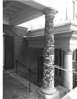
UNIVERSITY OF VIRGINIA Original brick column – cement plaster has been completely removed
