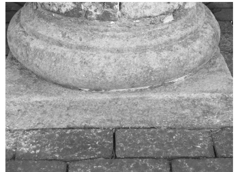
UNIVERSITY OF VIRGINIA Tuscan sand stone base after removal of coating and modern paints. Local sandstone was used to carve the original bases.
