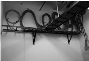
Structured cabling pathways and spaces
