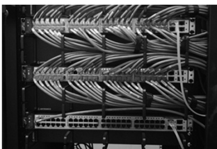
Category 6a cabling installed on Ethernet switch
