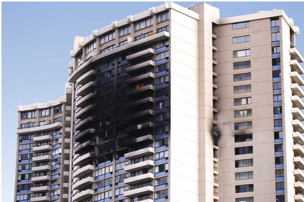
The charred exterior of the unsprinklered Marco Polo Building after in Honolulu, Hawaii, after a fire broke out in July 2017. Four people were killed in the fire. Kent Nishimura/AFP via Getty Images
