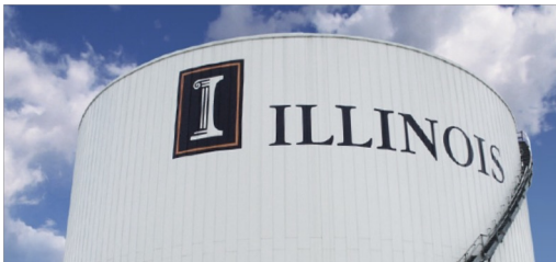
Thermal Energy Storage
