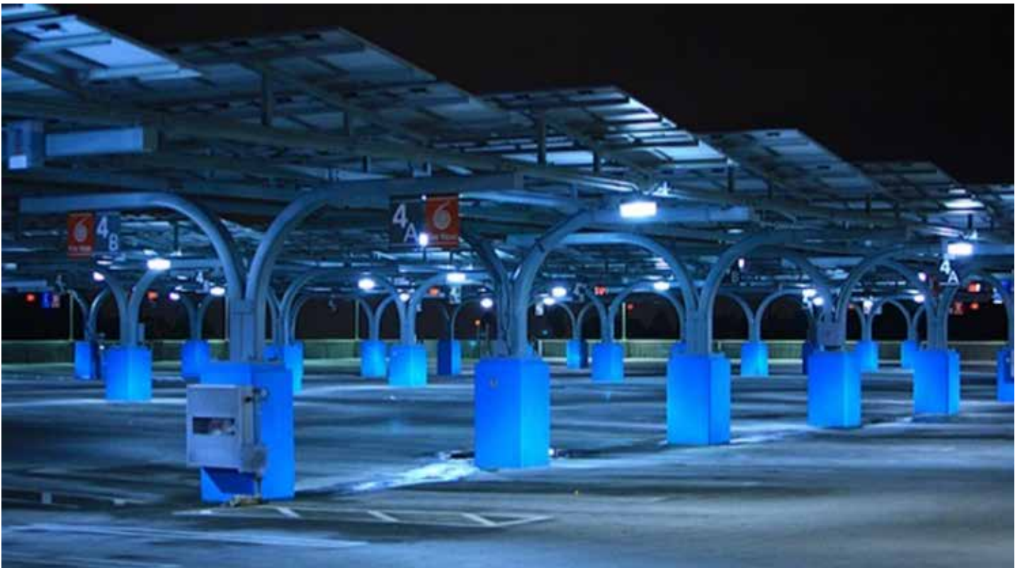
Solar Panels at Los Angeles Pierce College.
