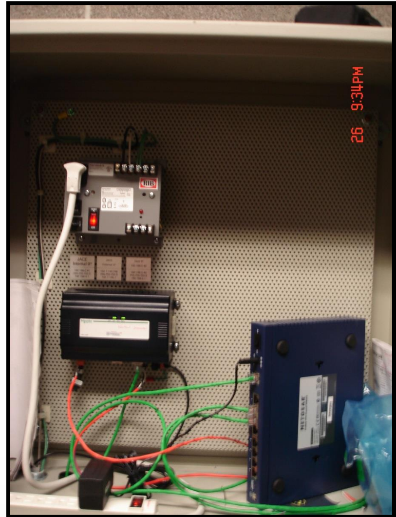
2 nd Gen Bldg Controller/Network
